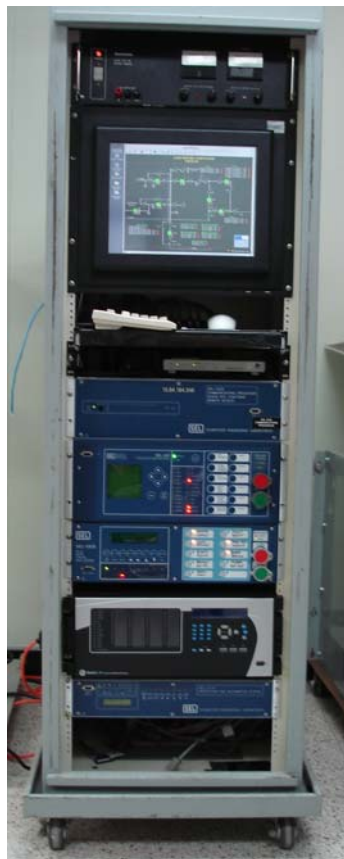
Figure 9. Portable Test Bed Used for Personnel Training
