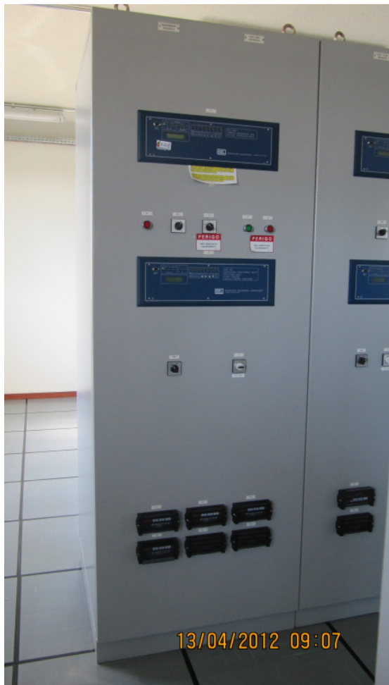
Figure 14: Copel protection panel
