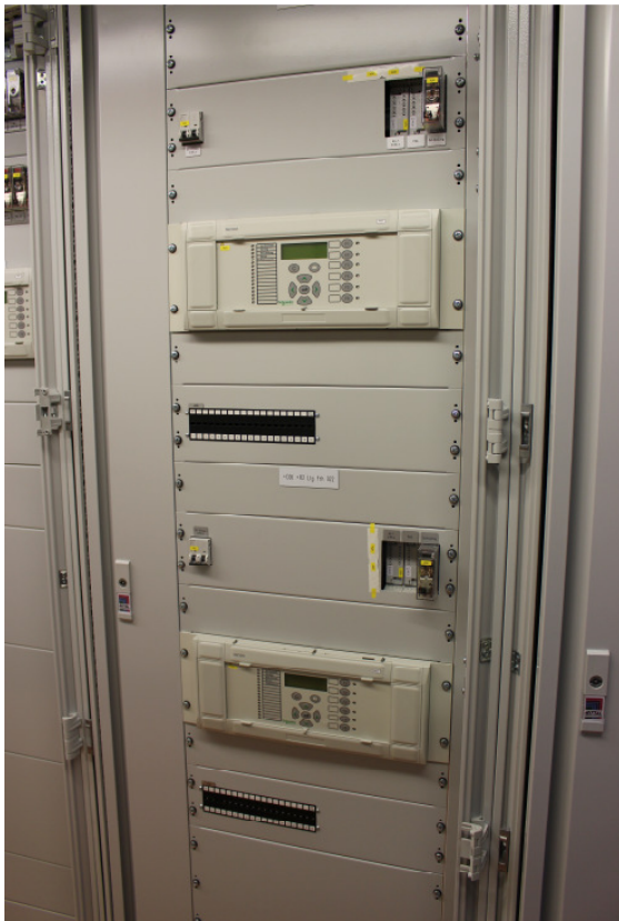
Figure 13: 50Hertz standardized protection panel for line differential protection
