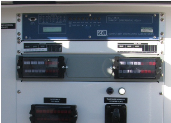
Figure 8: Example of a EKPC protection panel with standardized test access points
