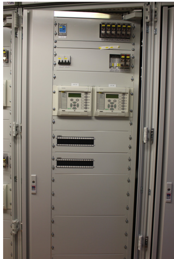
Figure 12: 50Hertz standardized protection panel for transformer protection
